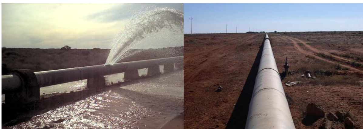
Figure 2 Menindee/Broken Hill pipeline burst
