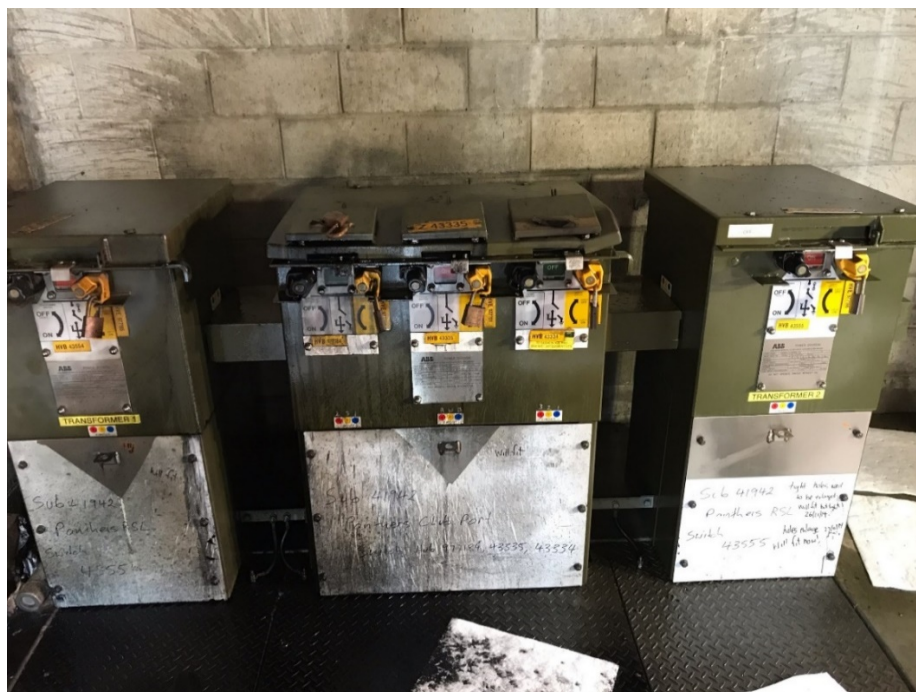
Image taken at site by a SafeWork NSW inspector after the accident
