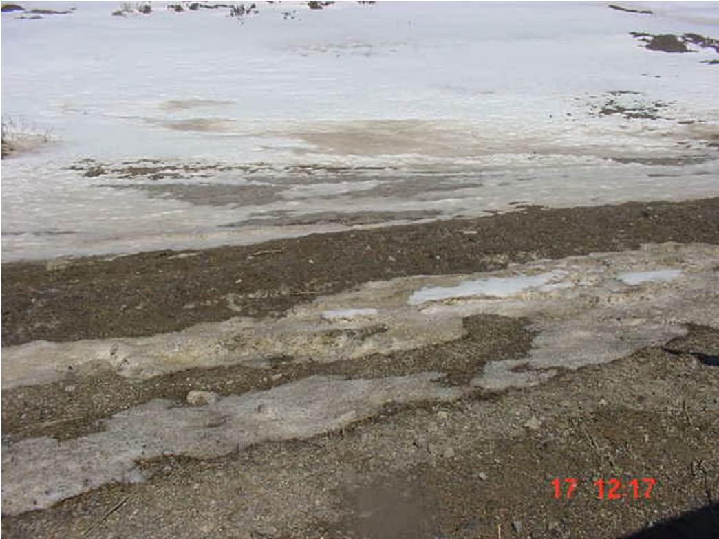
PHOTOGRAPH No.50. Gravel / dirt on snow alongside road and in creek from snow blowing.
