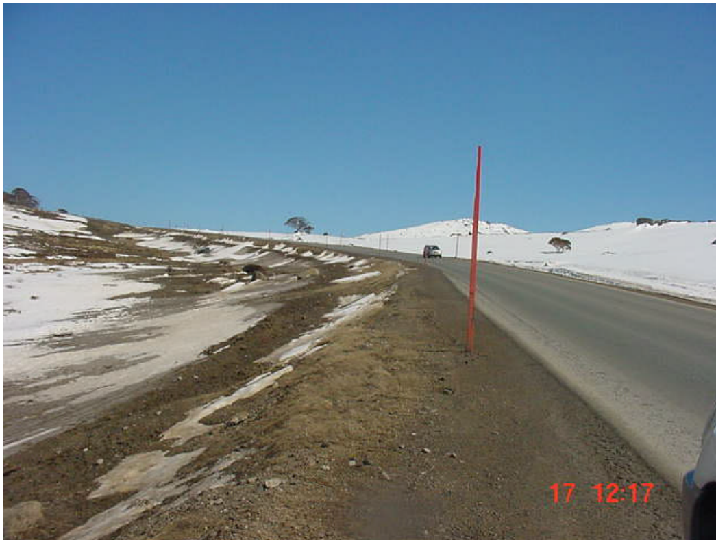
PHOTOGRAPH No.49. Kosciuszko Road – unsealed shoulder – effect of snow blowing on adjacent snow.
