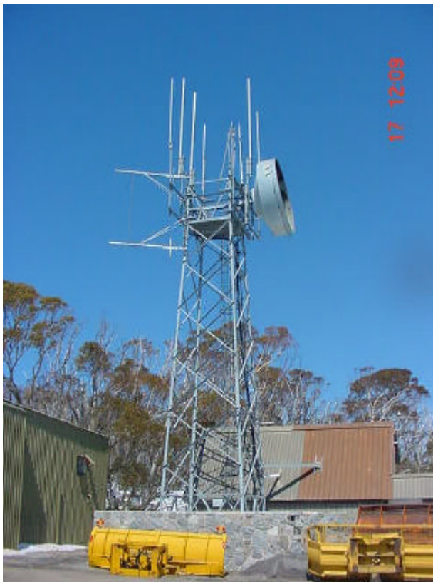
PHOTOGRAPH No.47. Communication tower / station at Smiggin Holes (workshop on left)
