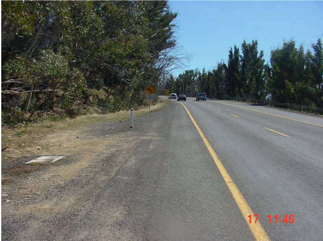
PHOTOGRAPH No.43 Kosciuszko Road –unsealed shoulder
