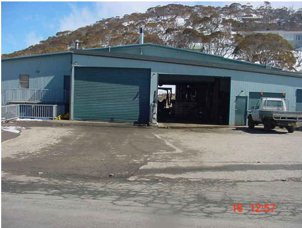
PHOTOGRAPH No.26. Smiggin Holes workshop (open petrol pump and contamination of asphalt)
