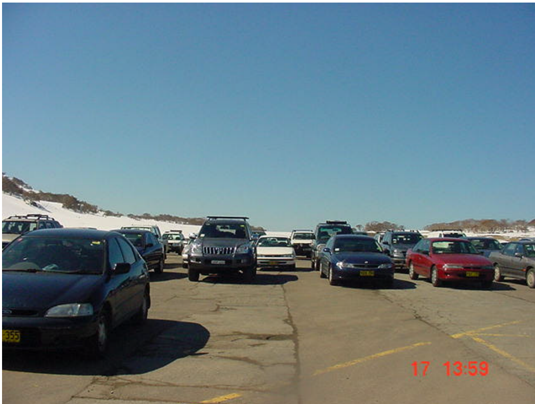
PHOTOGRAPH No.16. Example of scattered car parking (poor surface condition)
