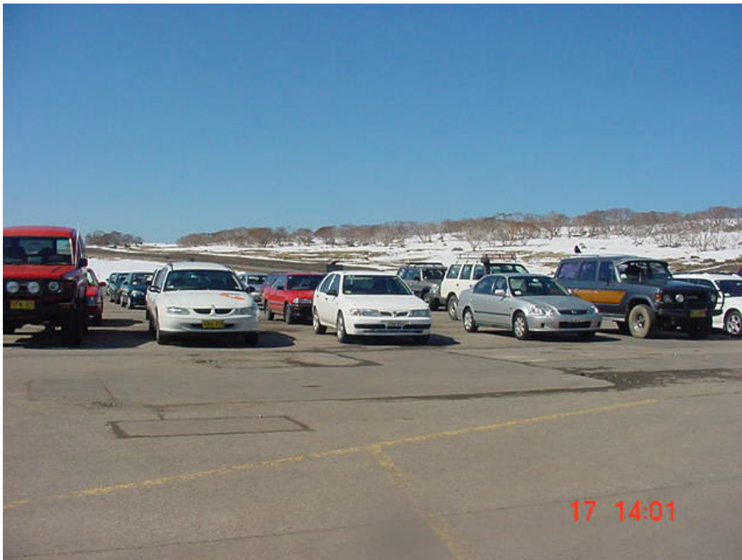
PHOTOGRAPH No.18. Another view of scattered car parking (poor surface condition)
