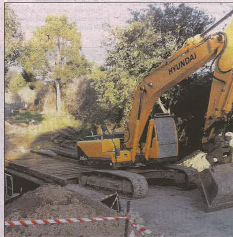
Funding is needed for bridges and roads: construction of Roses Rd Bridge
