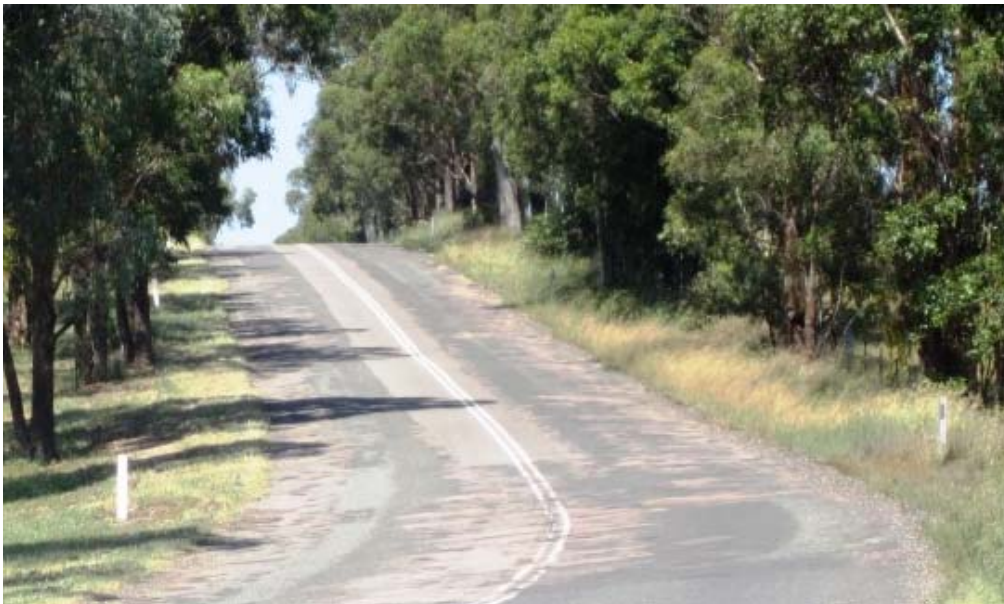
Failed – PCI less than 1.0
