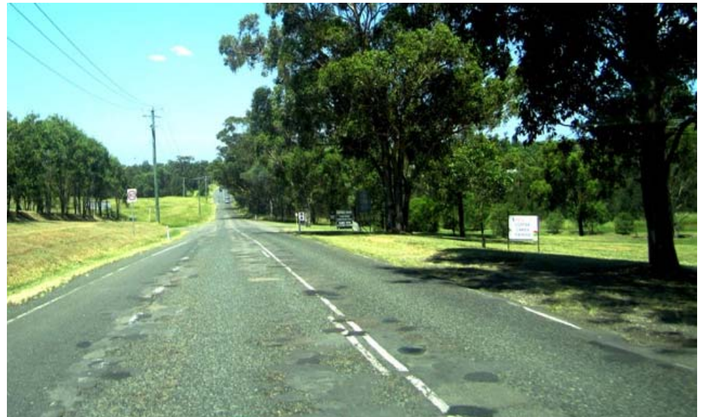
Failed – PCI less than 1.0
