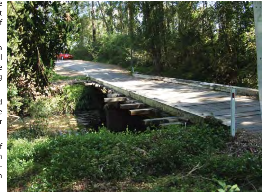
The bridge at Mill Creek Road, Stroud which currently has a load limit, will be replaced under the programme.
