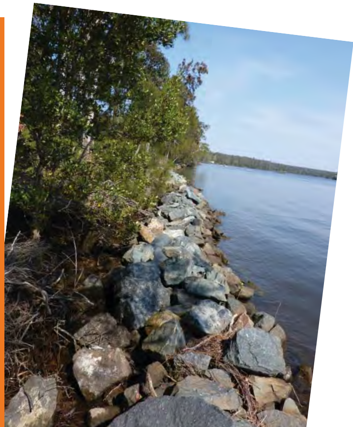
Construction of rock fillets and planting of native plants to ensure riverbank restoration.
