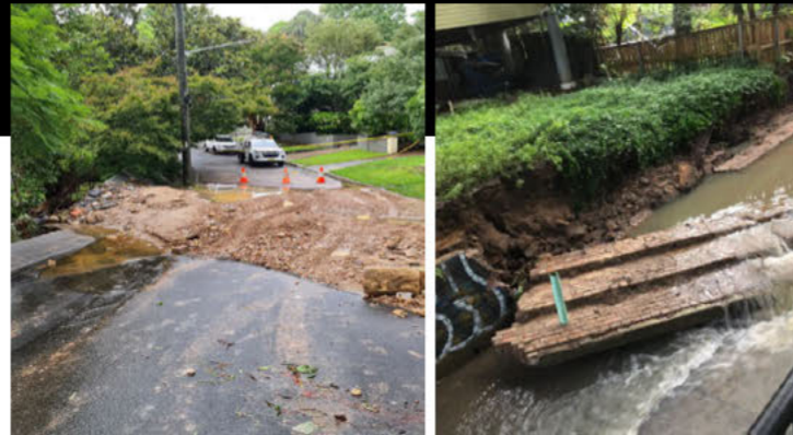
The Outpost, Northbridge Retaining wall collapse and stormwater pit blockage March 2022
