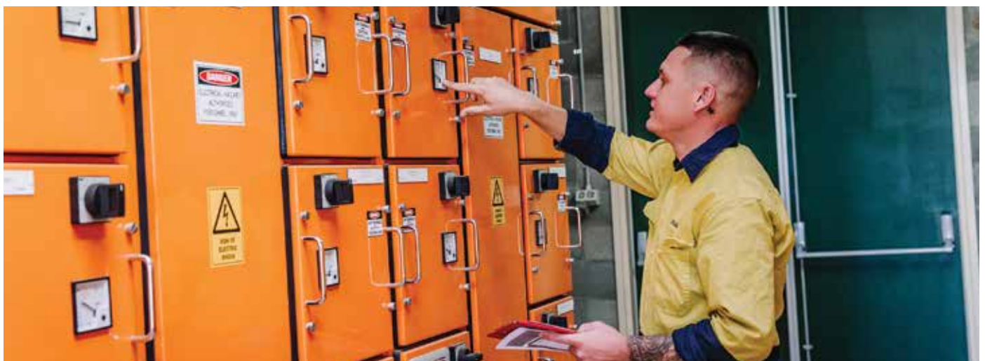
Westdale Water Treatment Plant
