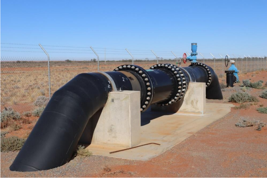
Figure 4 - Above ground pipeline
