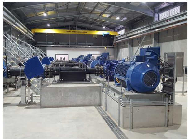
Figure 12 - WaterNSW pumping station
