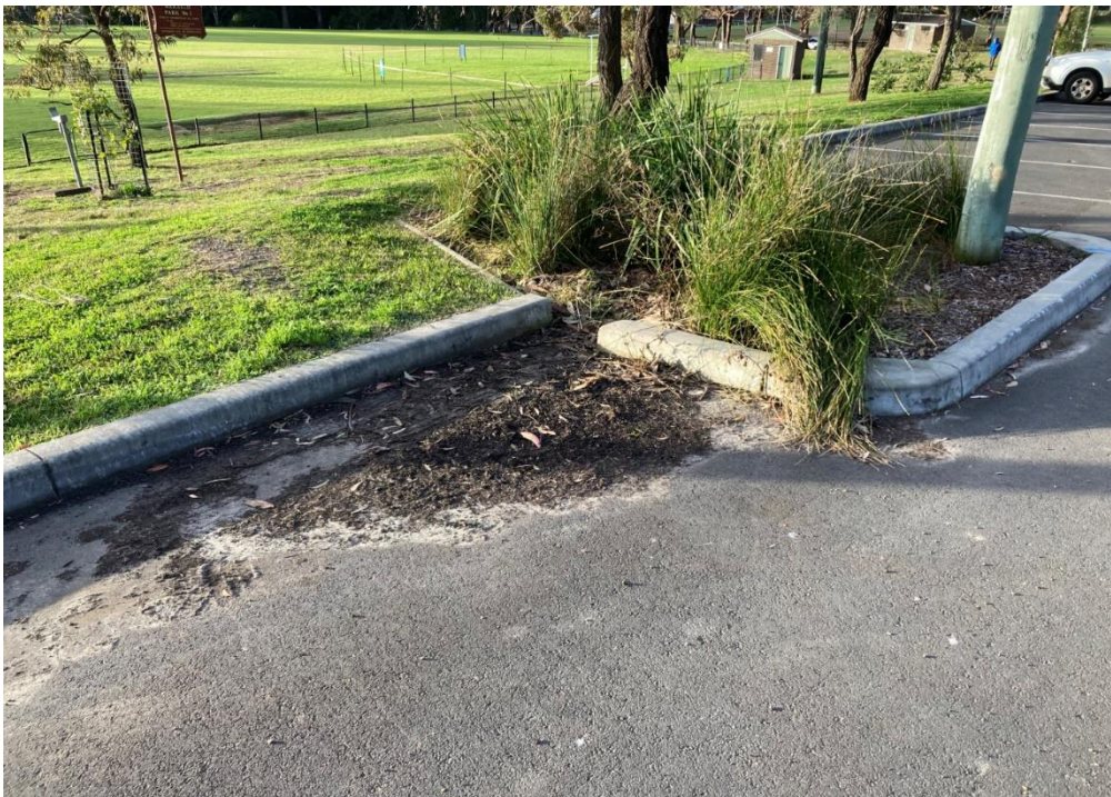
Figure 1 - Unmanaged Streetscape Raingarden
