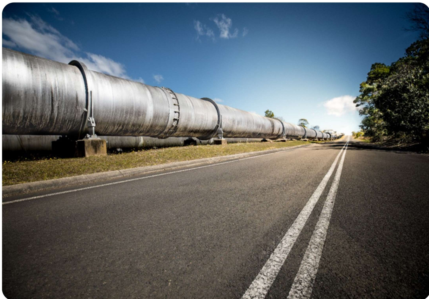
Figure 3 The trunk main that connects Prospect Reservoir to Warragamba Dam
