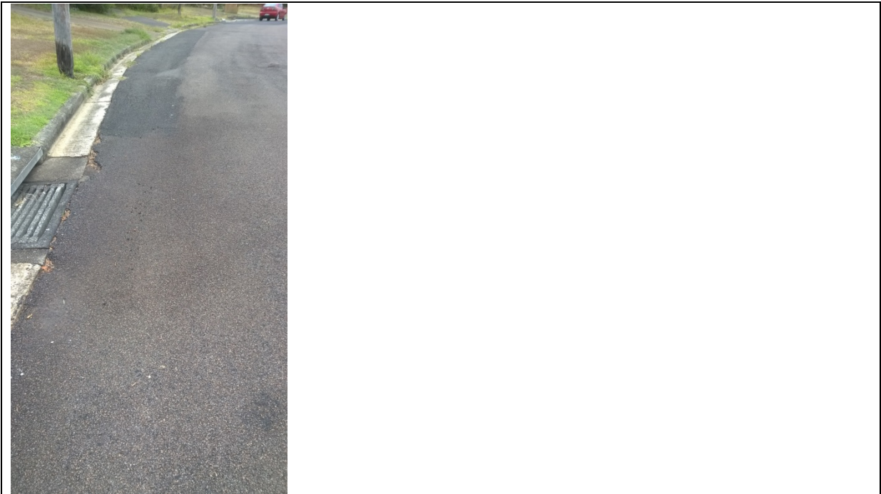
Pennington where section has not been repaired of new section
