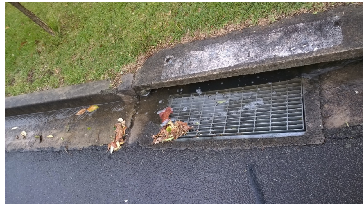
Alton Road Drain blocked
