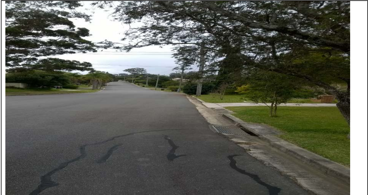
Alton Road gutter and road damaged
