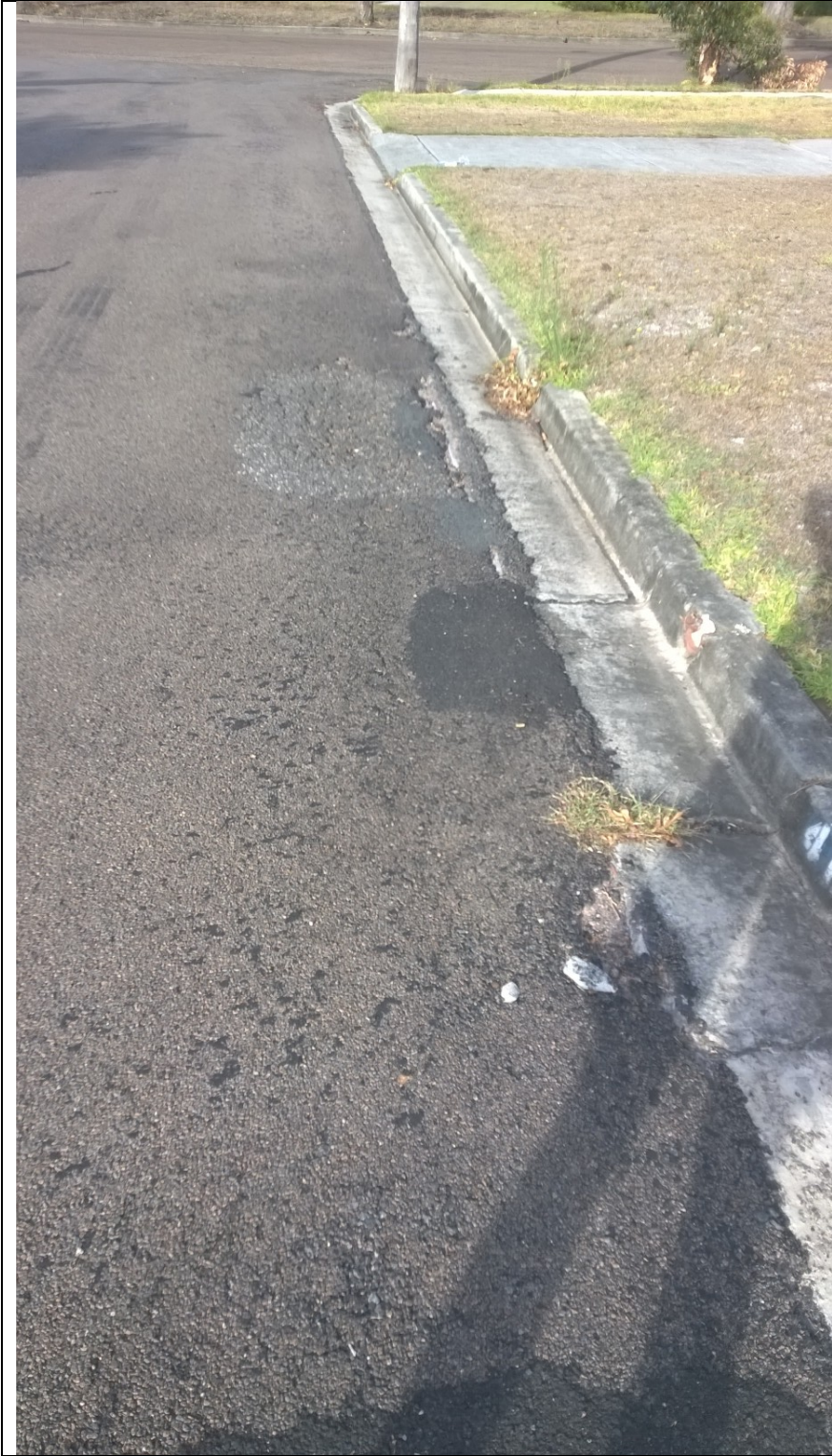
Pennington broken kerb and damaged tar
