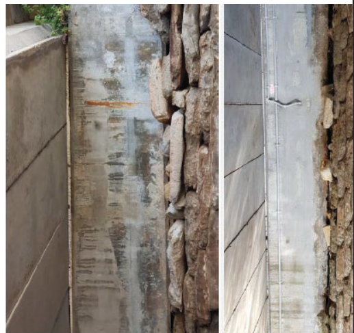
Photo No: 26 Abutment 2 Evidence of corrosion staining under unit 28.
