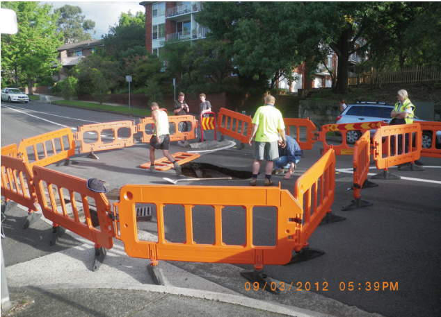
Sink hole in road near defective pipe
