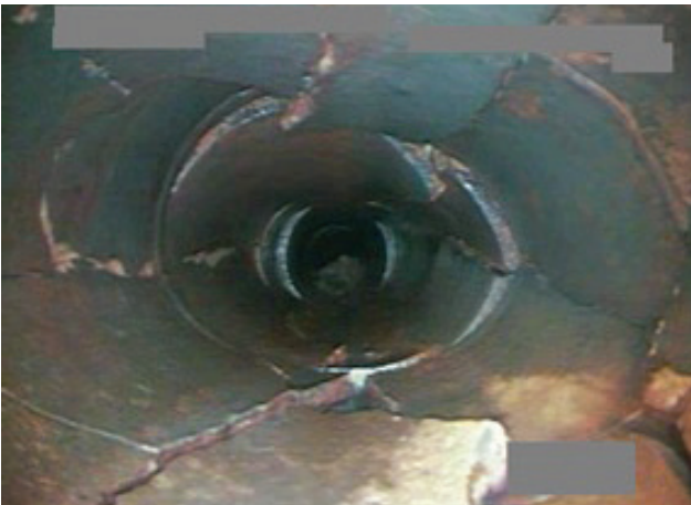
Pipe in very poor condition
