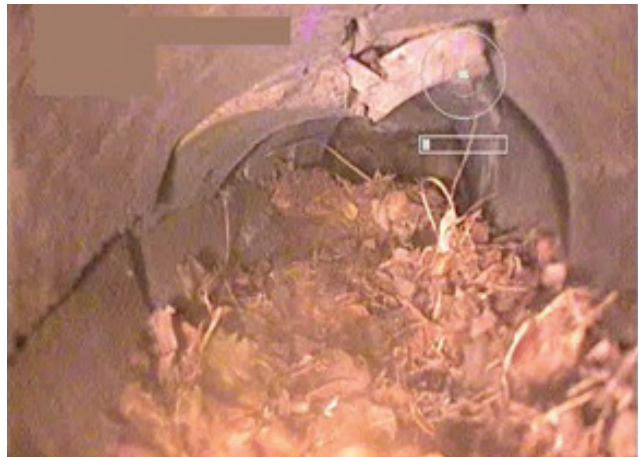
Pipe in very poor condition
