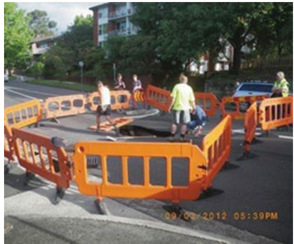
Sink hole in road near defective pipe
