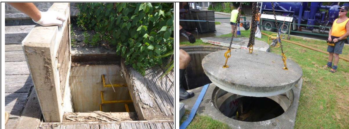
Lids are too heavy - The wood is starting to chip; they should be replaced. Lifting points rusted or broken off
