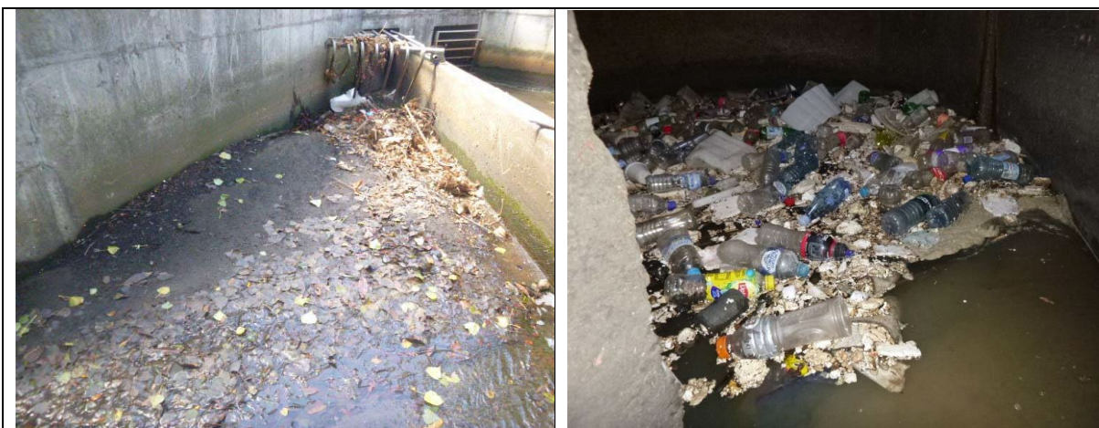
Sediment and trash build up in front of the weir and in pits generally – low capacity.
