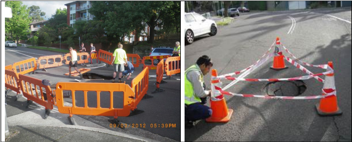
Sinkholes created from collapsed pipes and washout from leaking pipes
