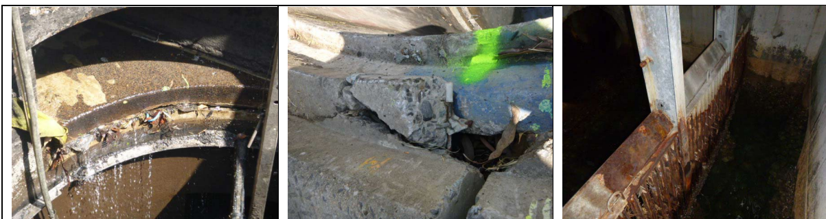
Corrosion and structural damage to GPT manhole covers
