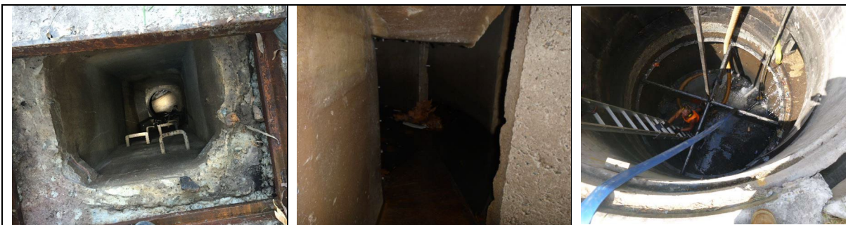
Difficult access to a lot of GPTs for maintenance
