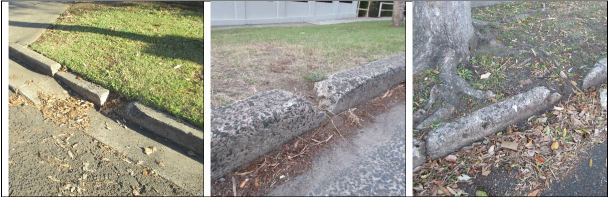
Examples of failed and failing Kerb and Gutter in the North Sydney LGA
