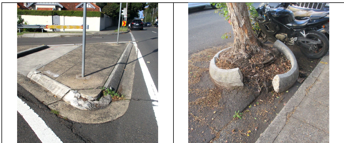
Examples of failed and failing Traffic Facilities in the North Sydney LGA
