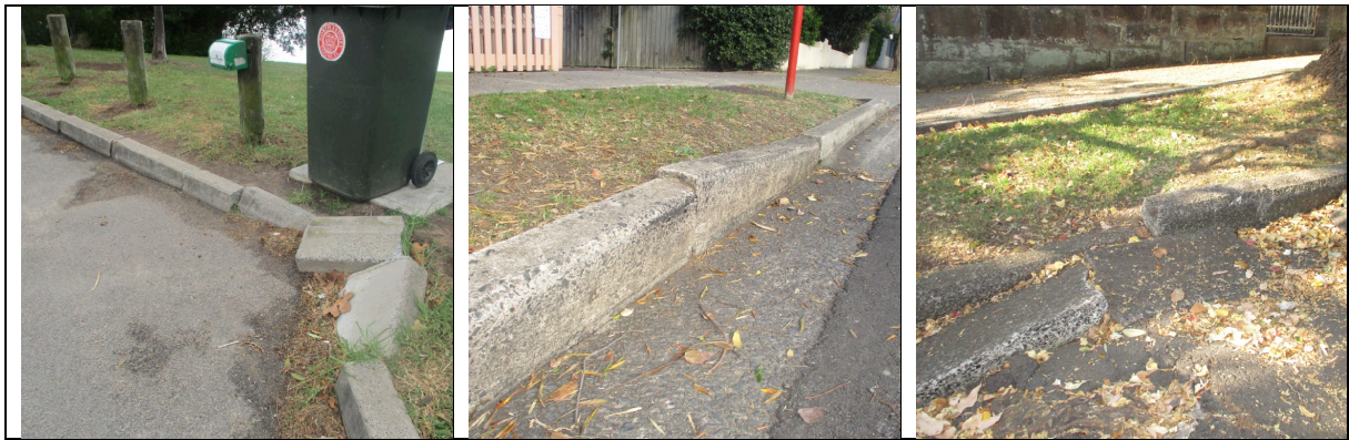
Examples of failed and failing Kerb and Gutter in the North Sydney LGA
