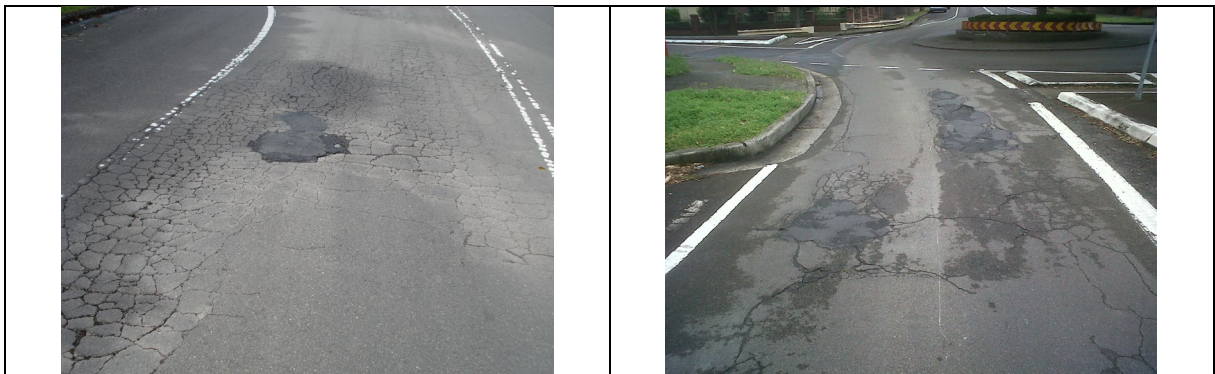
Examples of road pavements in poor condition in the North Sydney LGA
