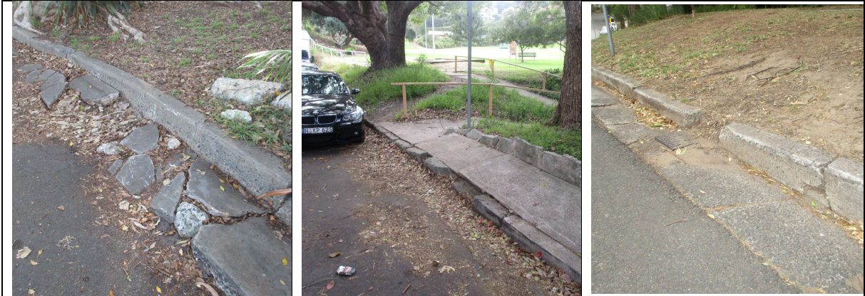
Examples of failed and failing Kerb and Gutter in the North Sydney LGA
