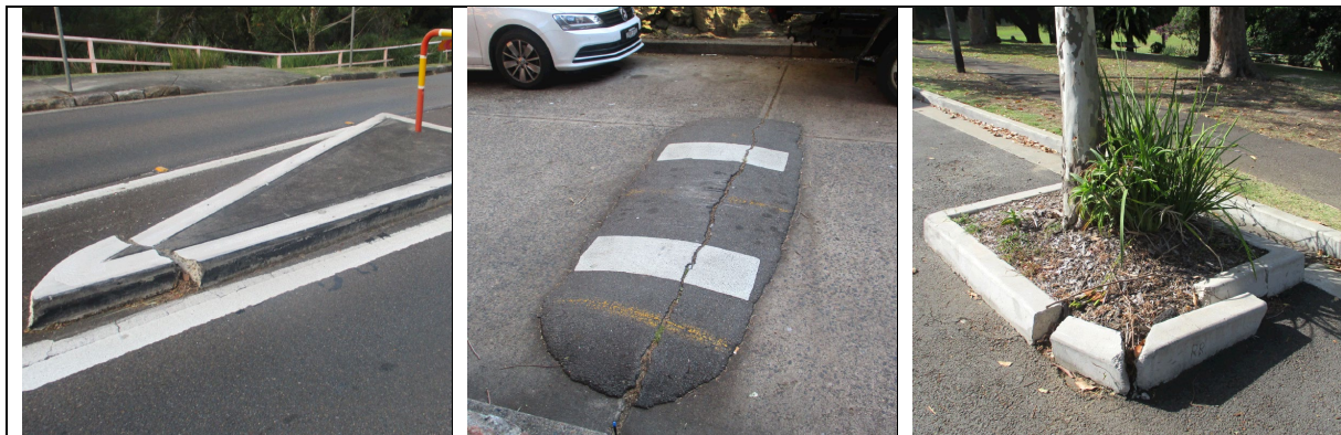
Examples of failed and failing Traffic Facilities in the North Sydney LGA
