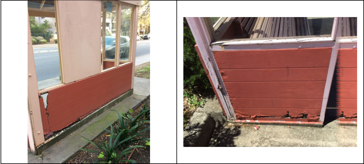
Examples of failed and failing Bus Shelters in the North Sydney LGA
