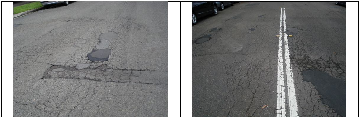
Examples of road pavements in poor condition in the North Sydney LGA
