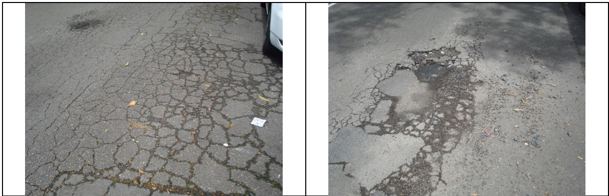
Examples of road pavements in poor condition in the North Sydney LGA
