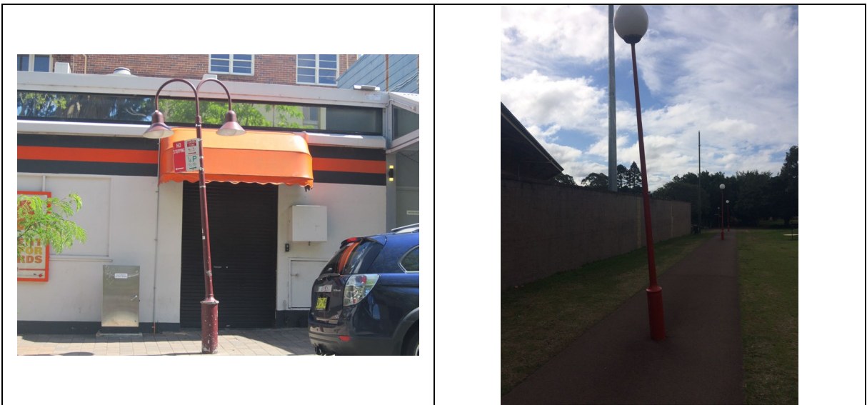
Examples of Lights in poor condition in the North Sydney LGA
