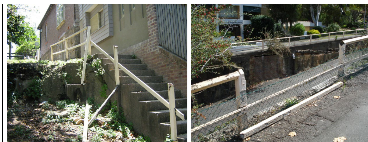
Examples of failed and failing Fences in the North Sydney LGA
