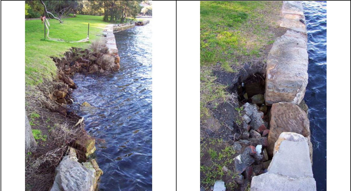
Examples of failed and failing seawalls in Sawmillers Reserve
