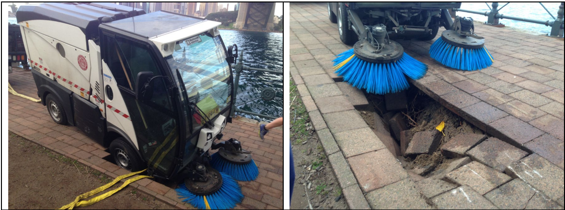
Examples of failed and failing seawalls in Bradfield Park
