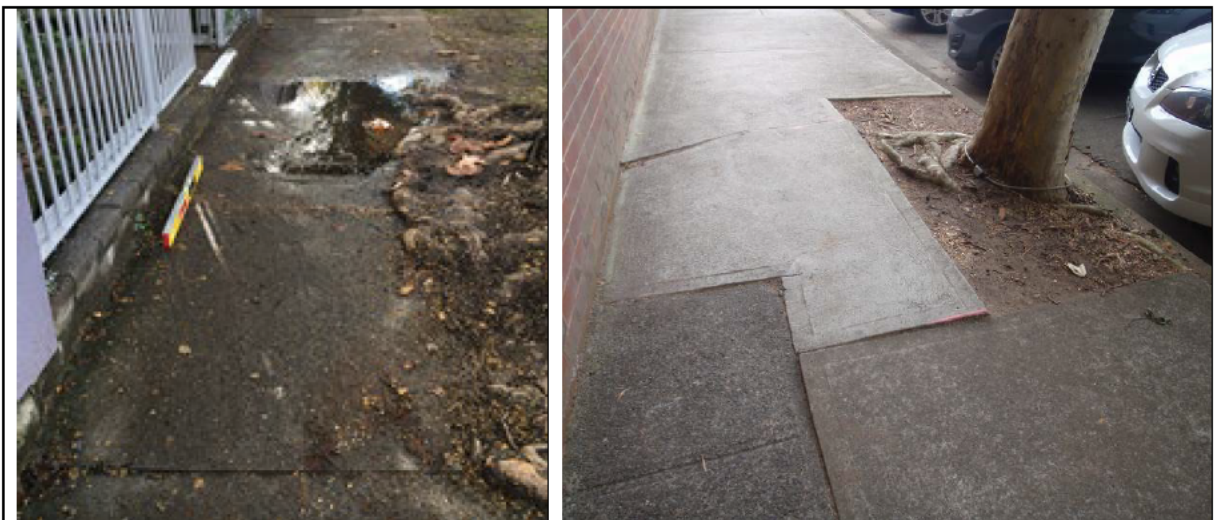
Tree root affected concrete footpath including ponding
