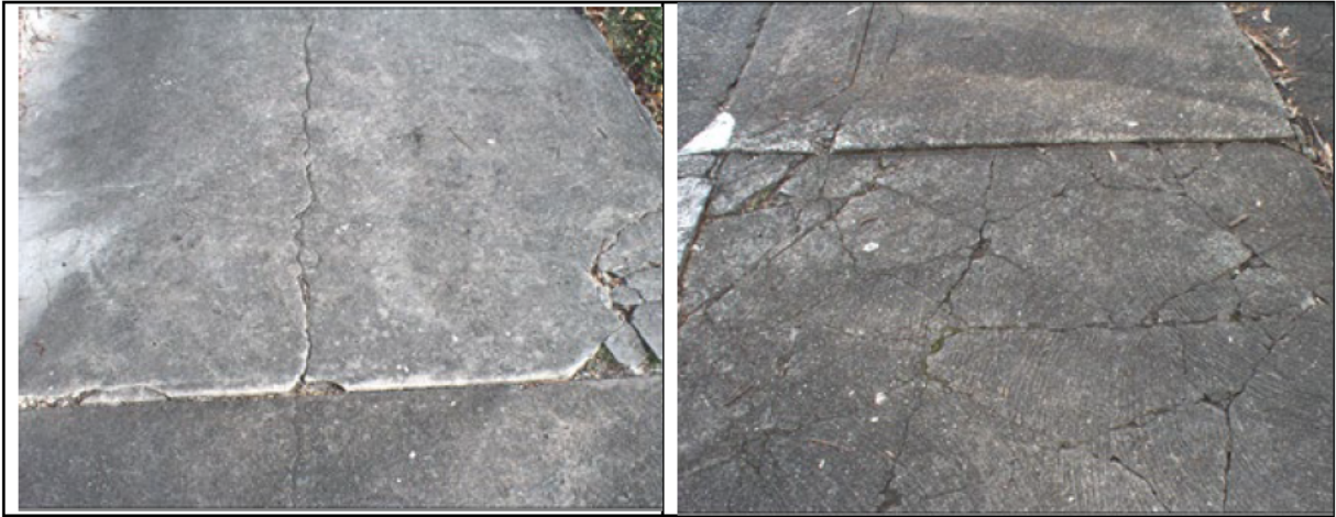
Concrete footpath in poor condition
