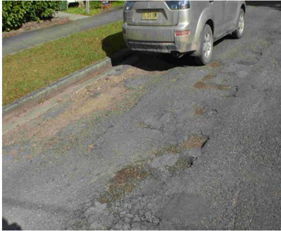
Example of a failed road pavement and damaged kerb and gutter
