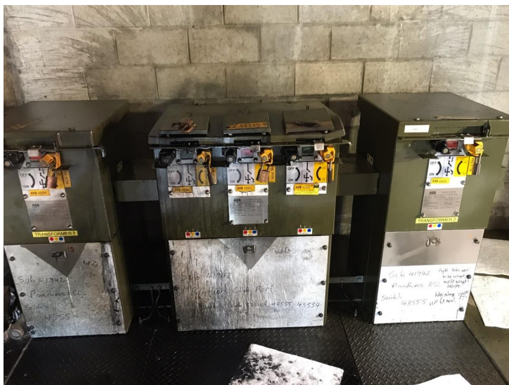
Image taken at site by a SafeWork NSW inspector after the accident
