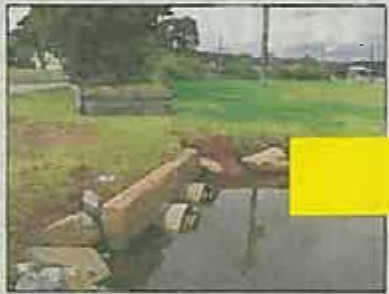
FLAT FLAPS: The two drainage pipes at Quota Park with one-way flaps are not enough to drain off water after a heavy downpour, according to some.
