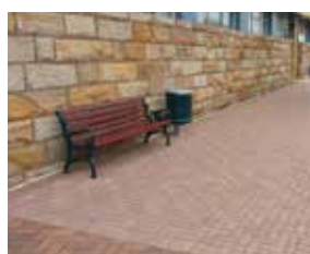
RENEWAL OF FOOTPATH, KERB AND GUTTER, SEATS AND BINS AT THE MITTAGONG PLAYHOUSE.
