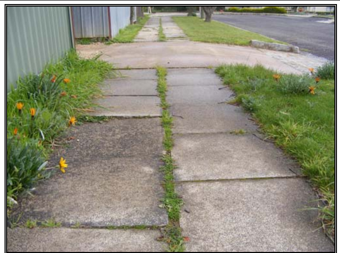
Condition 6 Extensive movement
