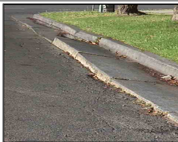
Condition 9 Extreme movement and lack of Function
