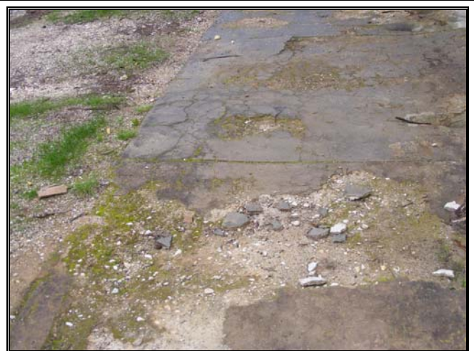
Condition 9 Very poor Condition – Cracking and breaking up
