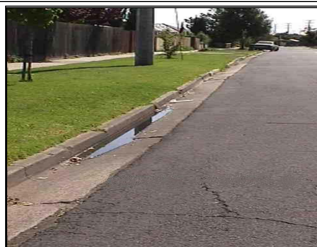
Condition 8 Large movement and holding of water
