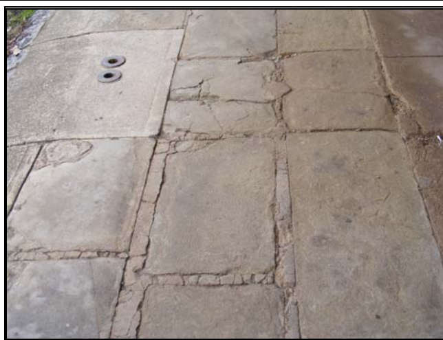
Condition 7 Extensive cracking and movement
