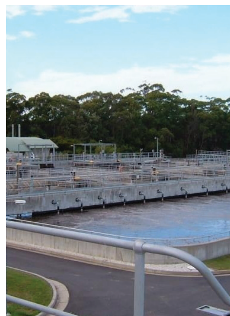
Banora Point Waste Water Treatment Plant
