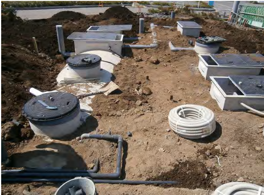
Image 2: Configuration of Wastewater Tanks
