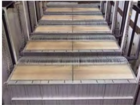
Submerged Membrane Unit (MBR)
