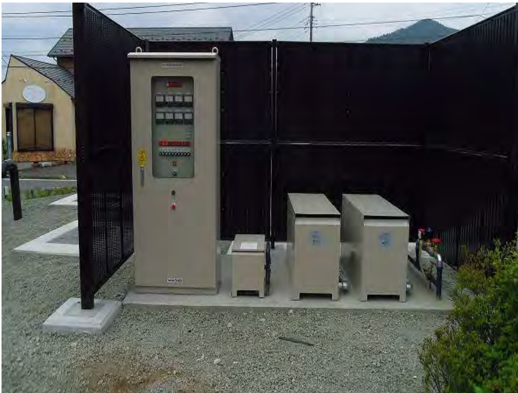
Image 4: Control Boxes for Wastewater Tanks
