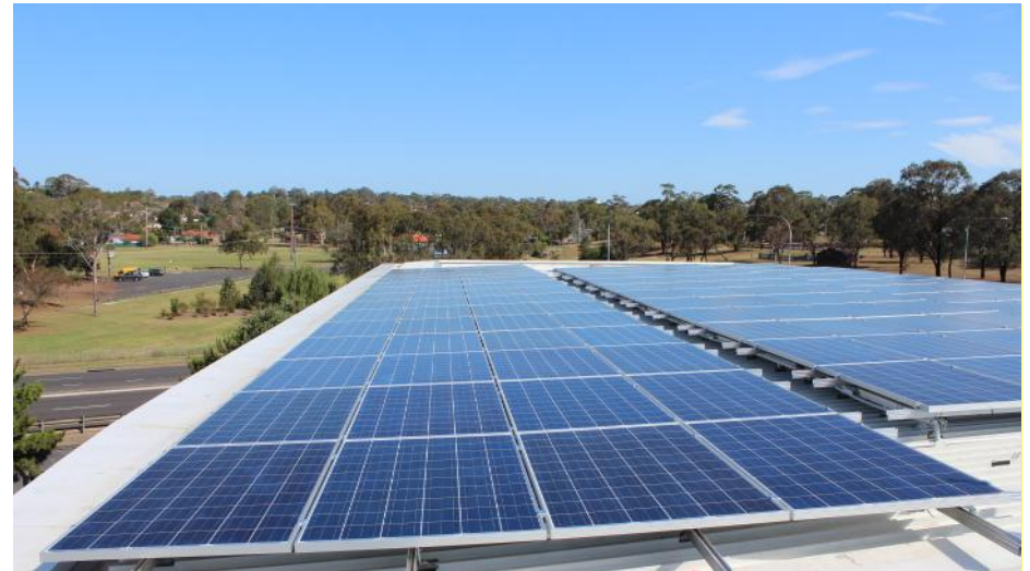
(Campbelltown Arts Centre – solar panel sustainability initiative)
