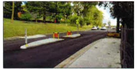
UPDATE: Council recently completed the installation of a new pedestrian crossing refuge in South West Rocks.
