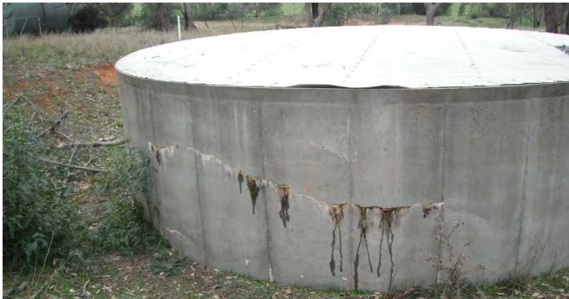
Figure 2: Active cracking, Little Brocklesby Reservoir
