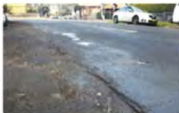
Condition 4 - Denman Avenue, Summer Hill
