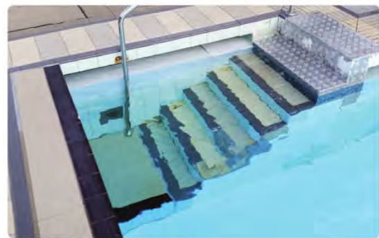
Pool steps that are collapsing
