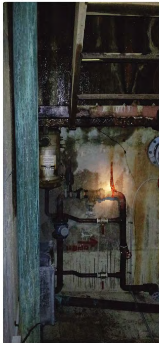
Old outdoor pipe-work
