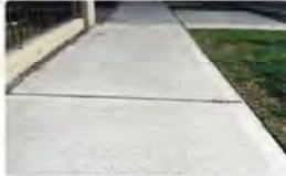
Condition 1 - Hillcrest Avenue, Ashfield
