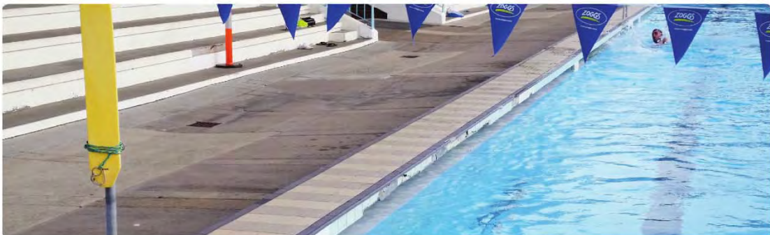
Concrete cancer on the pool tiles
