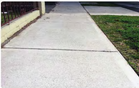
Condition 1 - Hillcrest Avenue, Ashfield
