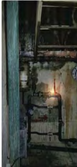
Old outdoor pipe-work
