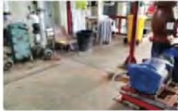
Old pool pumps
