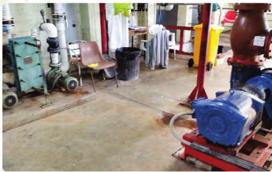
Old pool pumps
