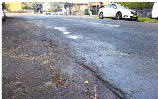
Condition 4 - Denman Avenue, Summer Hill
