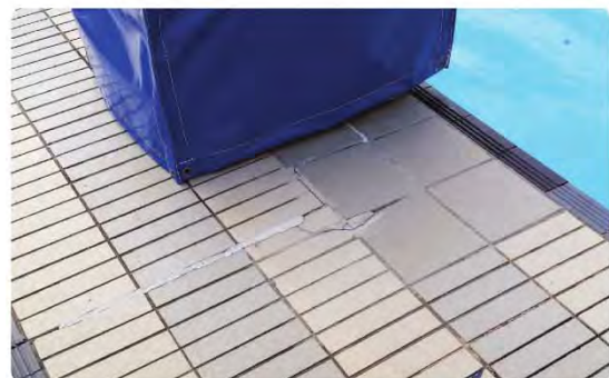
Pool edge which is collapsing from concrete cancer
