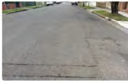
Condition 3 - Carshalton Street, Croydon
