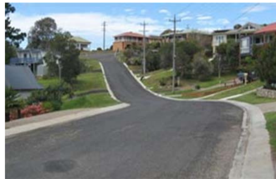
Road Reconstruction program which achieves a renewed urban road often with drainage improvements such as Hadrill Parade, Dalmeny shown above before & after reconstruction 2009
