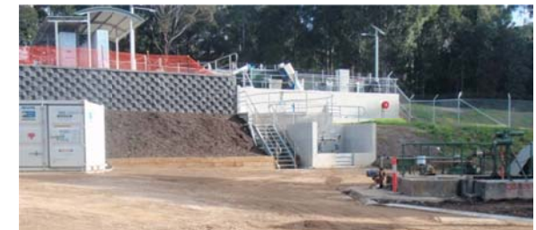
The new Batemans Bay Sewage Treatment Plant inlet works prior to completion
