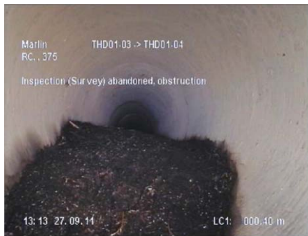
Stormwater pipe blocked with tree roots-condition monitoring image September 2011
