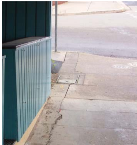
Example of the type of footpath backlog maintenance & renewal work which needs attention (pictured main street Narooma)
