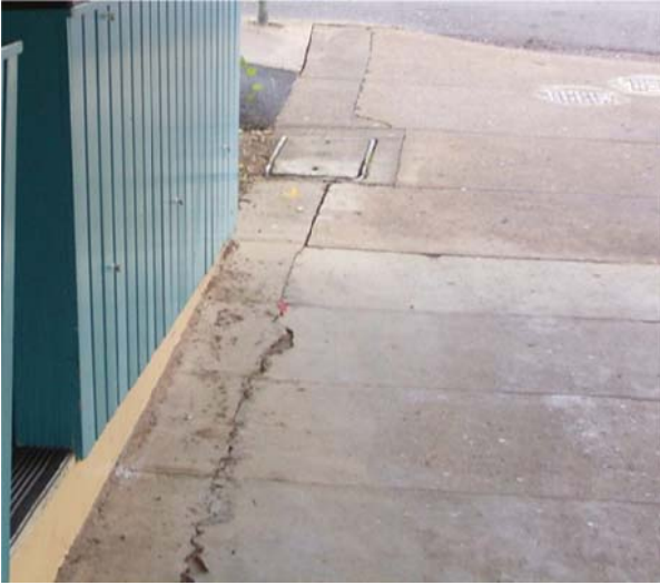
Failing footpath requiring attention
