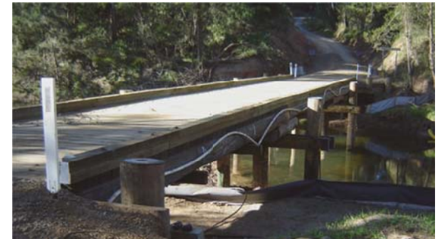
Cadgee Bridge before & after renewal- adding many years to the life of the bridge
