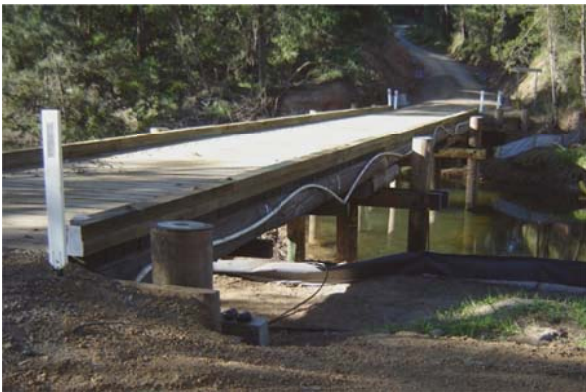
Bridge renewal is an example of the critical infrastructure we need to maintain and renew. Pictured above is Cadgee Bridge on Eurobodalla Road before and after renewal works in 2011 which will add 20 years to the life of girders, providing a vital link to rural areas.
