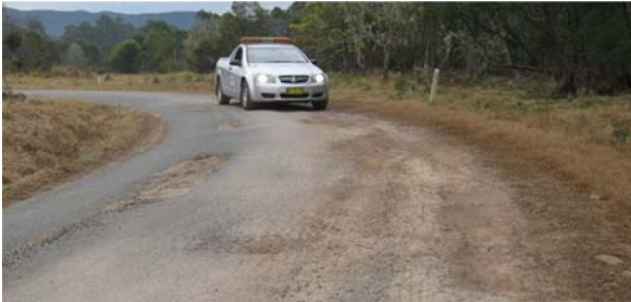
A rural road now too far gone for resealing, requiring rehabilitation - an example of rehabilitation backlog that would be addressed under Scenario 3
