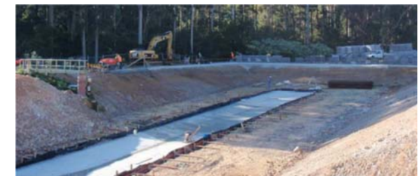
The storm detention pond at the Batemans Bay Sewage Treatment Plant during construction
