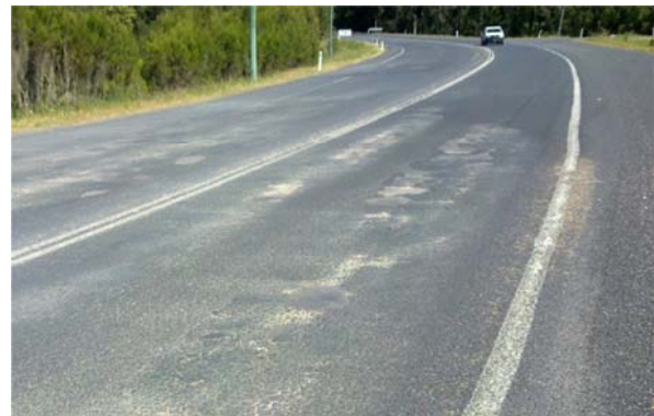
Pavement condition deterioration accelerates during wet weather, an example above of work required on George Bass Drive near Glenella Rd.
