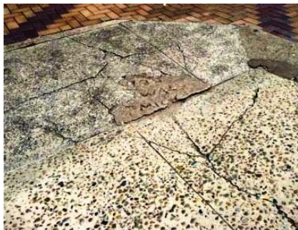
Path in "fair" condition
