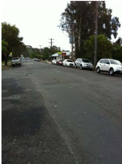
Road in "fair" condition
