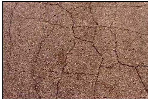
Condition 5 – Very poor
