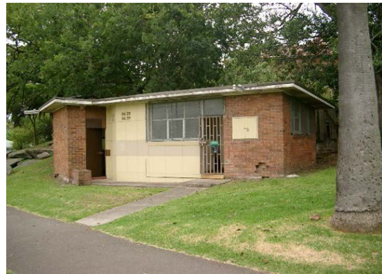
Condition 5 – Very Poor
