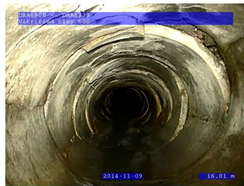
Condition 5 – Very Poor
