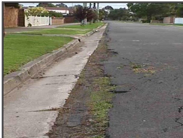
Condition 6 Movement and concrete breakdown
