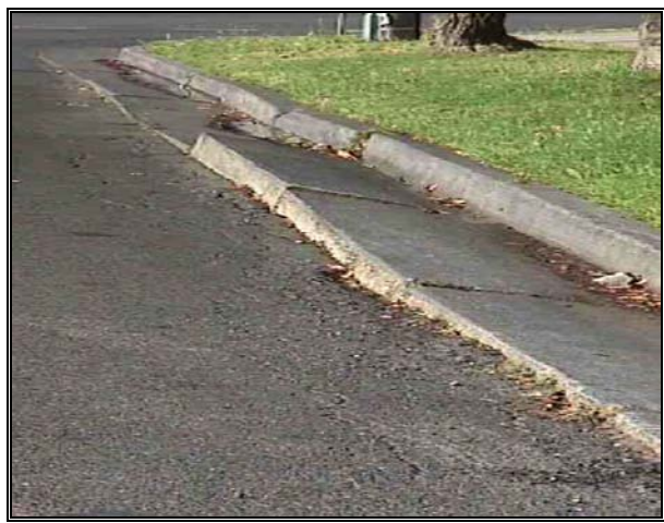
Condition 9 Extreme movement and lack of function
